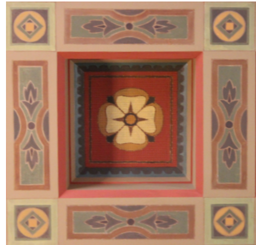
Ceiling Restoration Project - Los Angeles Union Station J.Dunbar as Senior Project Architect for Architectural Resources Group Completed in 2017
