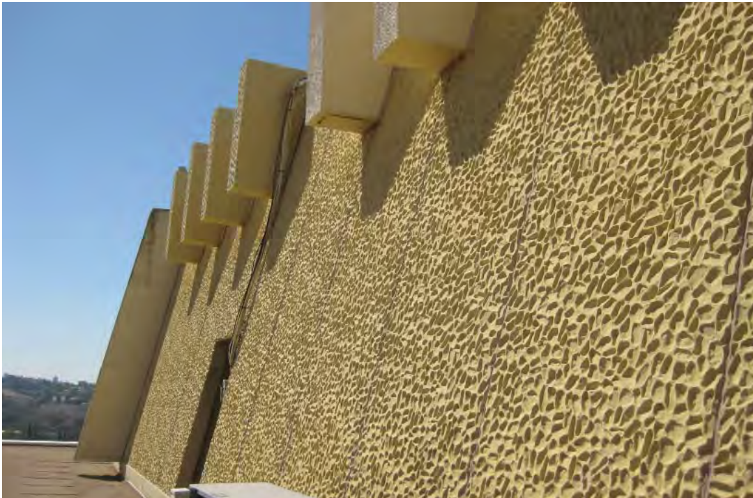
Image 42: The sixth floor roof. Textured fiberglass fins have been added to conceal some of the added equipment on the upper edge of the roof.
