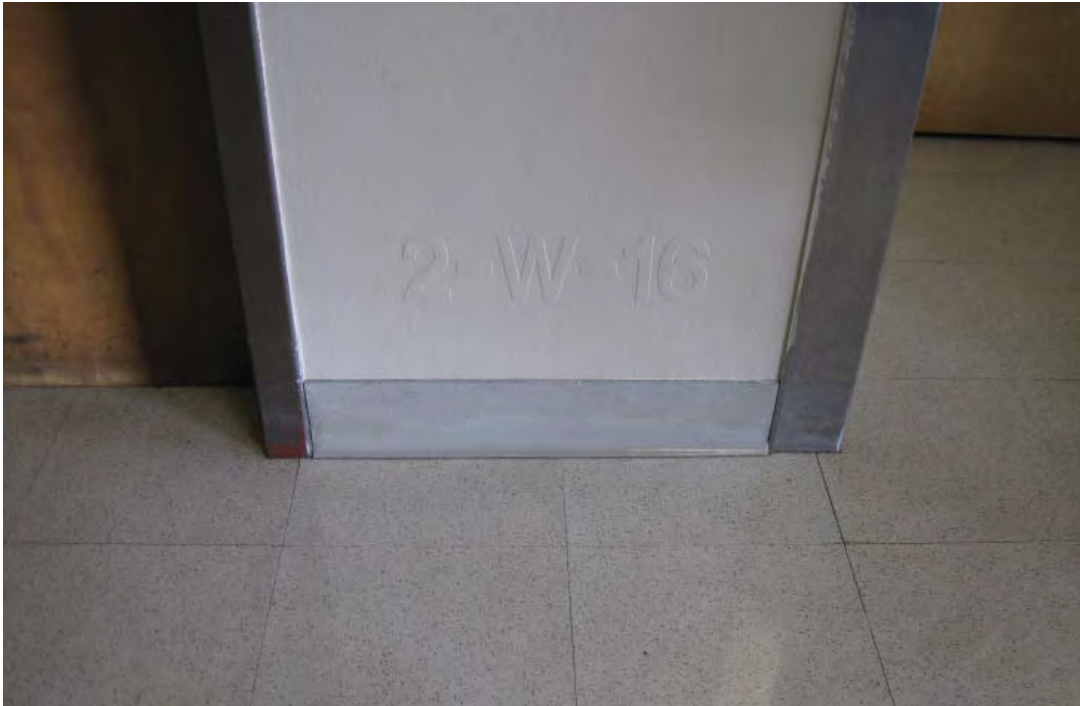
Image 30: A numbered structural column. The numbers corresponds with the original drawings and can be found on structural columns throughout the building.
