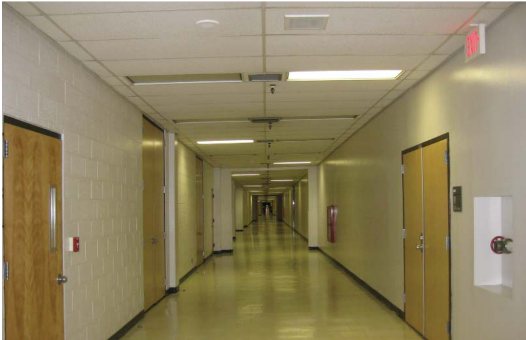
Image 24: A typical interior corridor on the first floor. The suspended ceiling is original and matches interior photos from the 1970s (Refer to Image 5).
