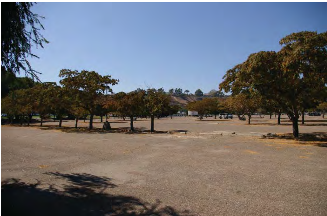
Image 21: The southwest corner of the parking area. The outer sections of parking are under utilized and not regularly maintained.
