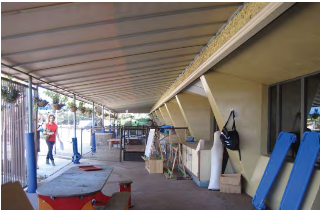
Image 37: The child care center on the third floor. A new sheet metal shade canopy has been added on the original exterior wall.
