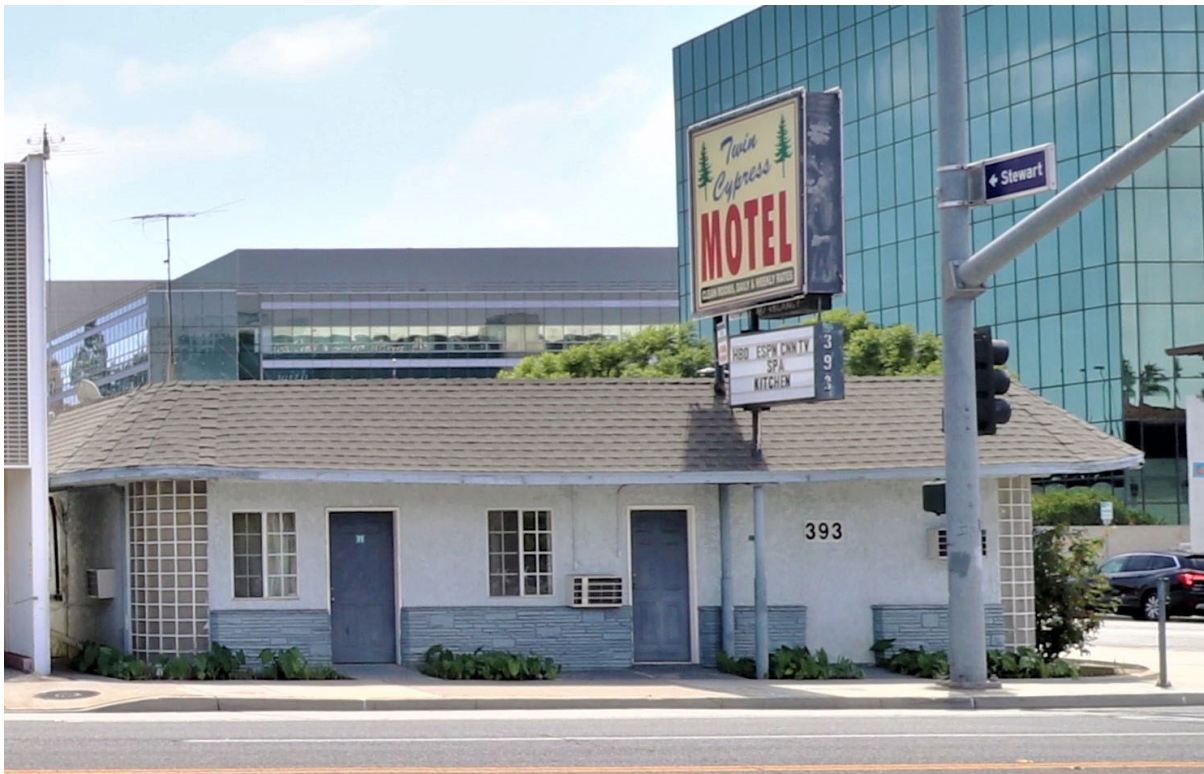
Figure 12: West elevation of the Twin Cypress Motel, view to the east (6/4/2020). Note missing door where street numbers are and the relocated pole sign.
