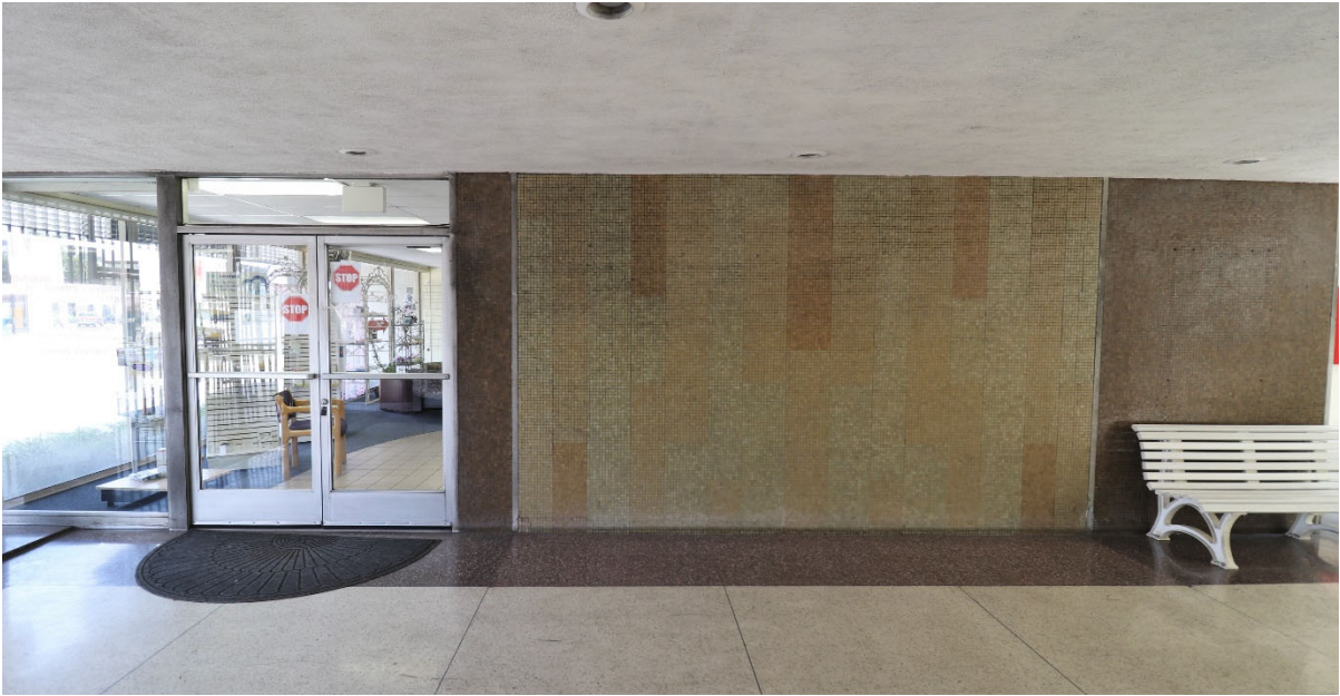
Figure 8: Terrazzo floor, mosaic tile wall, and aluminum-framed storefront. View to the north (6/4/2020).
